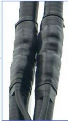
Seal the joint points (three layers of waterproof tape + three layers of insulation tape)
