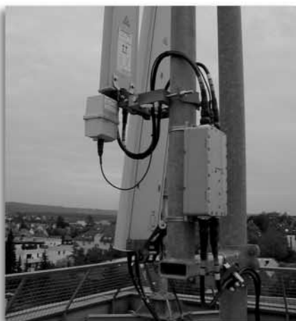
UMTS site of the operator Vodafone in Germany with Kathrein's RET system.
