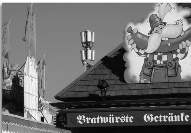
UMTS site of the operator T-Mobile at the "Oktoberfest" in Munich (Germany) with Kathrein's RET system.
