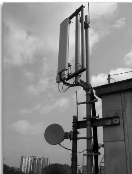
UMTS site of the operator Centertel in Poland with Kathrein's RET system.
