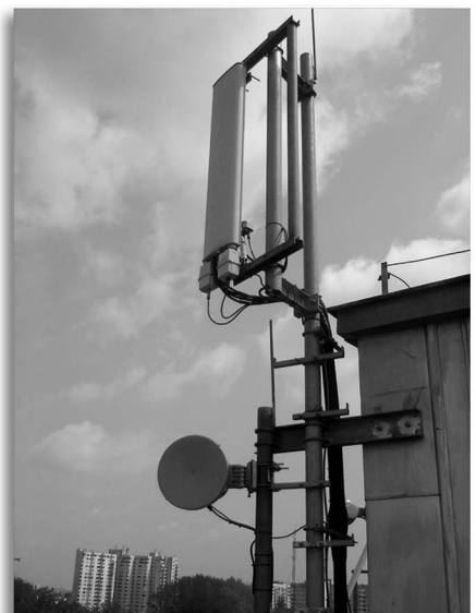
UMTS site of the operator Centertel in Poland with Kathrein's RET system.
