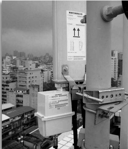
UMTS site of the operator THC in Taipei (Taiwan) with Kathrein's RET system.
