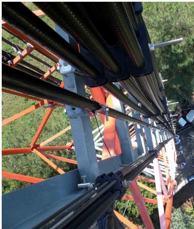
Top: Six corrugated coax cables for 3 sectors
