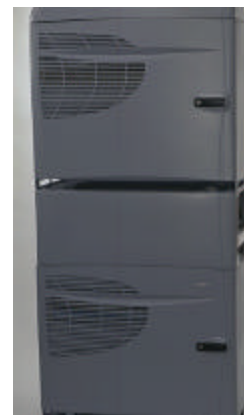
Two Vertically stacked Horizon Indoor BTS cabinets
